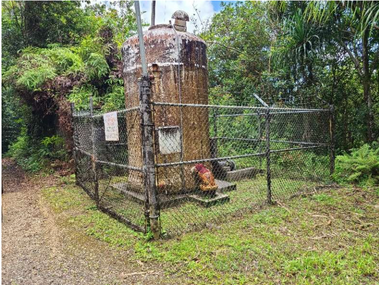
21. HHFDC State Well Site – Surge Tank
